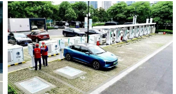
State Grid Hangzhou Xiaoshan Asian Games Village Charging Station
